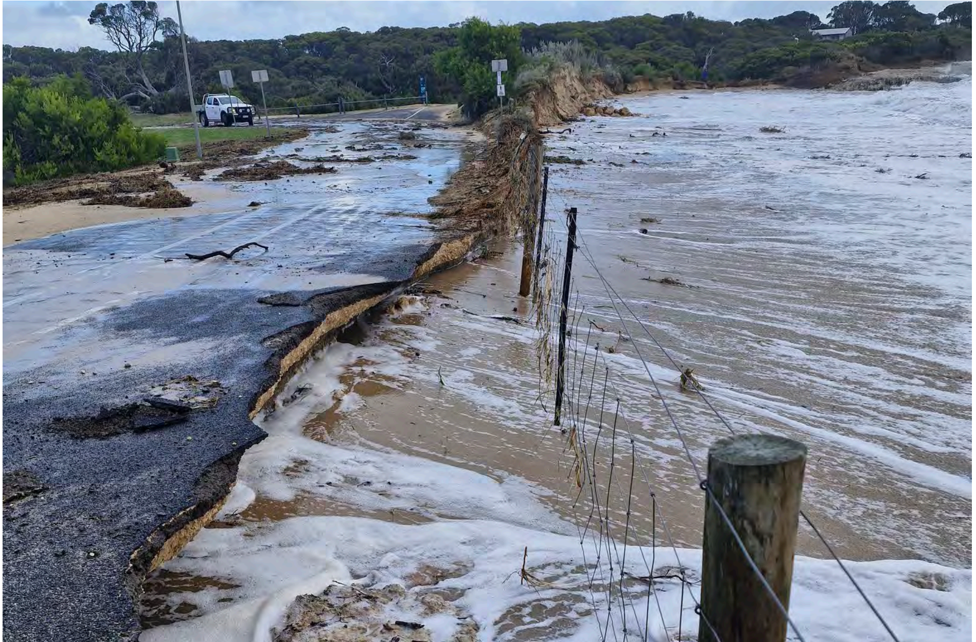
Image 10: Storms in 2025 resulted in significant erosion on beaches along the Limestone Coast, including in Robe. Pictured is a road behind Fox Beach in Robe, which was damaged by flooding and erosion.
