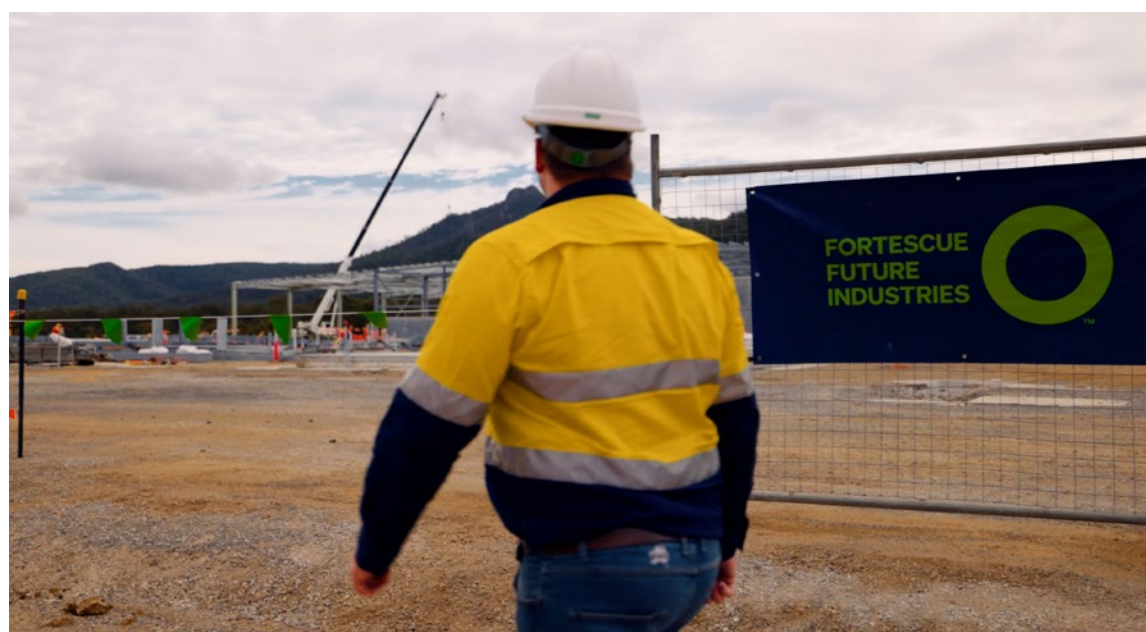
Figure 13: In February 2022, construction began on Fortescue Future Industries' (FFI) Green Energy Manufacturing Centre in Gladstone, Queensland. Once completed, it will help meet growing green hydrogen demand, which reached an estimated 87 million metric tons (Mt) in 2020, and is expected to grow to 500–680 Mt by 2050 (World Bank 2022).
