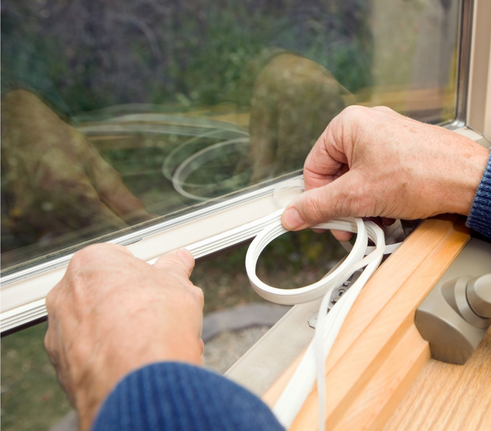
Image 3. Major savings: Installing readily available and affordable seals to windows is one method of reducing draughts, which can mean major savings on bills.
