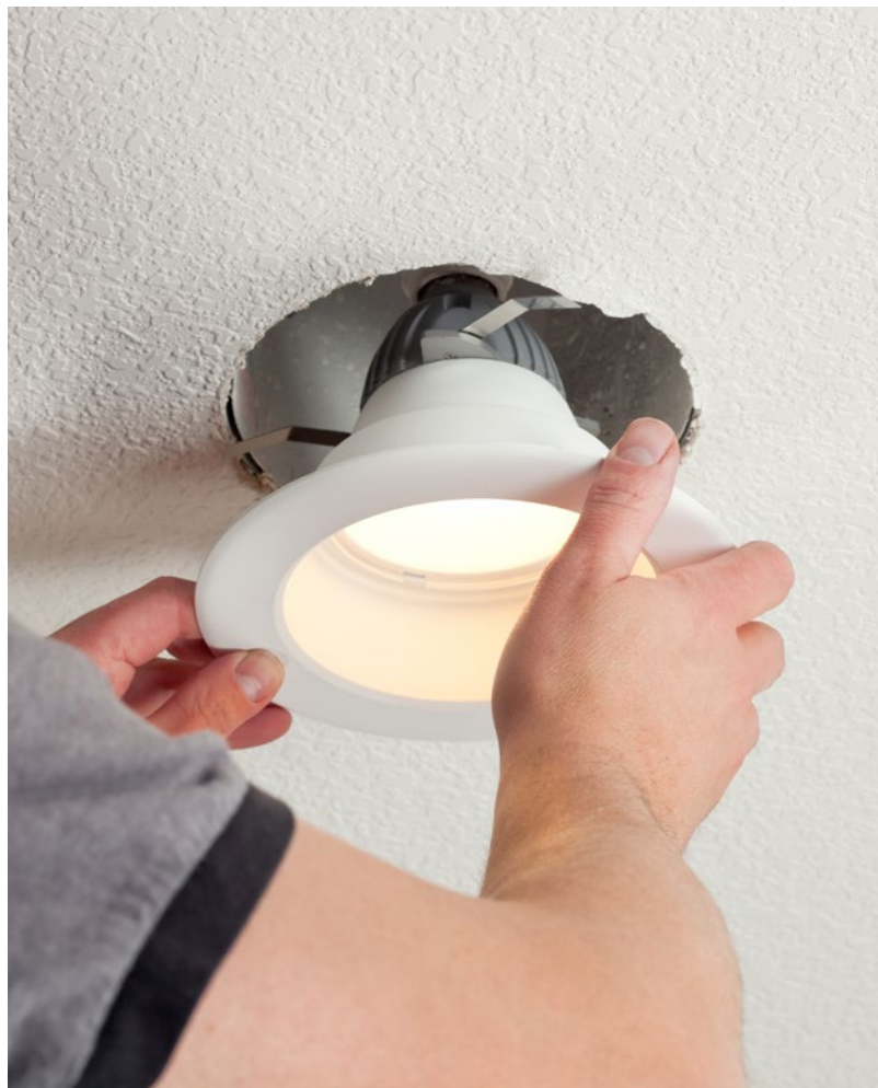
Image 1. Smarter lighting: Installing LED globes or replacing halogen downlights with LEDs can save up to 80 percent of lighting electricity costs.
