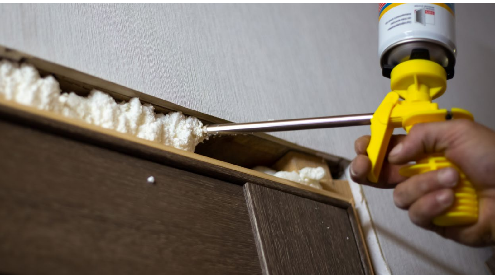
Image 4. Readily-available: Filling large gaps is important for draught proofing and can be done using expanding foams that are readily available at hardware stores.
