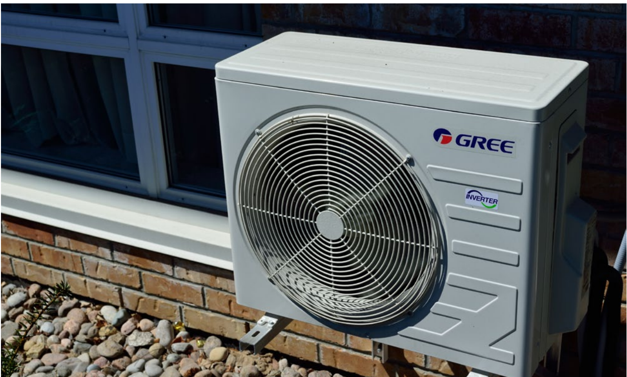
Figure 3: Air source heat pumps are the most common type of heat pump. The number installed in Australia has continued to increase over the years, from 7,822 in 2015 to 31,094 in 2020 (Statistica 2022).
