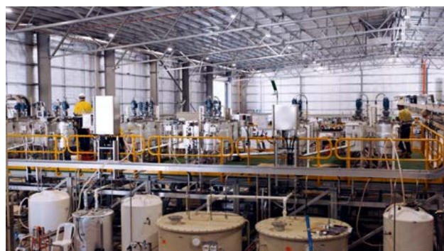
Figure 12: Alpha HPA’s new industrial site at Gladstone. This facility will be one of the largest single HPA refineries in the world. The International Aluminium Institute (2022) predicts global aluminium demand will increase by almost 40 per cent by 2030. Alpha HPA’s aluminium will be key to meeting this growing demand, while also supporting our journey to net zero.
