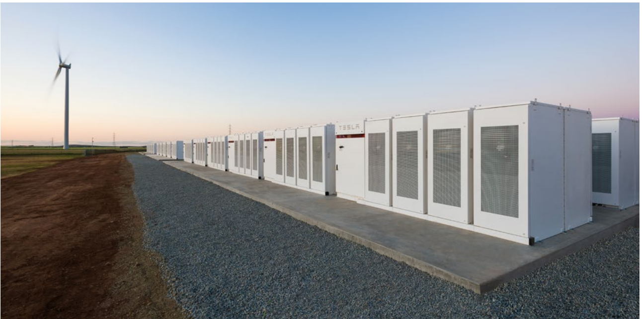
Figure 4: The Hornsdale Power Reserve in South Australia is the world's first big battery and was the largest lithium-ion battery at the time of installation in 2017. A mandatory Renewable Energy Storage Target would help ensure that sufficient storage is supplied.
