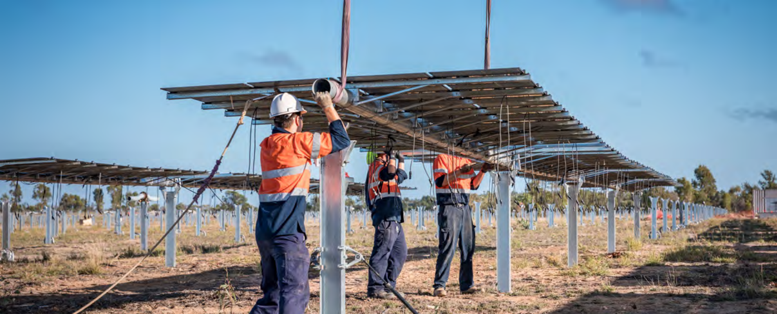
Figure 6: Workers install the Kidston Solar Project in Far North Queensland. The renewable energy industry could support more than 11,000 jobs in Queensland by 2025 with strong policy support.
