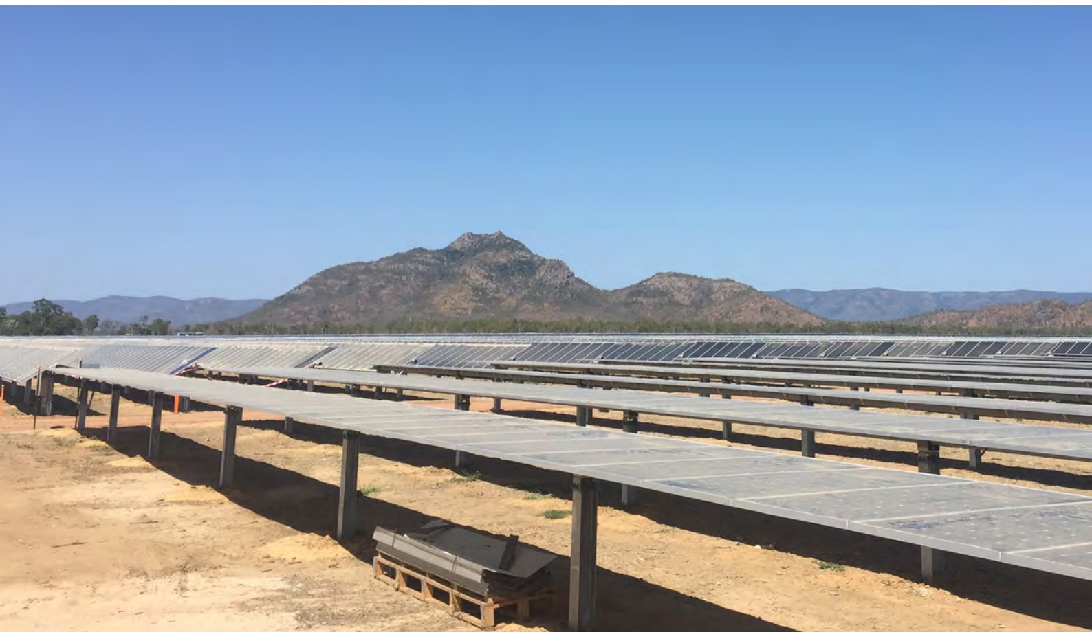
Figure 4: REZs will help drive down power bills and spur job creation throughout Queensland. (Pictured: Ross River Solar Farm near Townsville).
