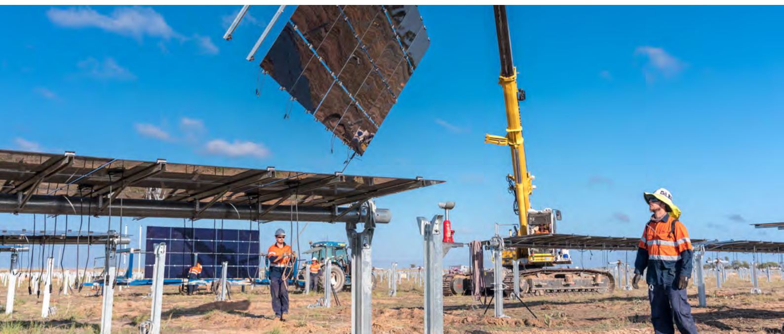
Figure 10: Queensland has a competitive advantage in renewable energy and can lead in harnessing renewable energy for job creation and economic growth. (Pictured: Workers at Kidston Solar Project in Far North Queensland).
