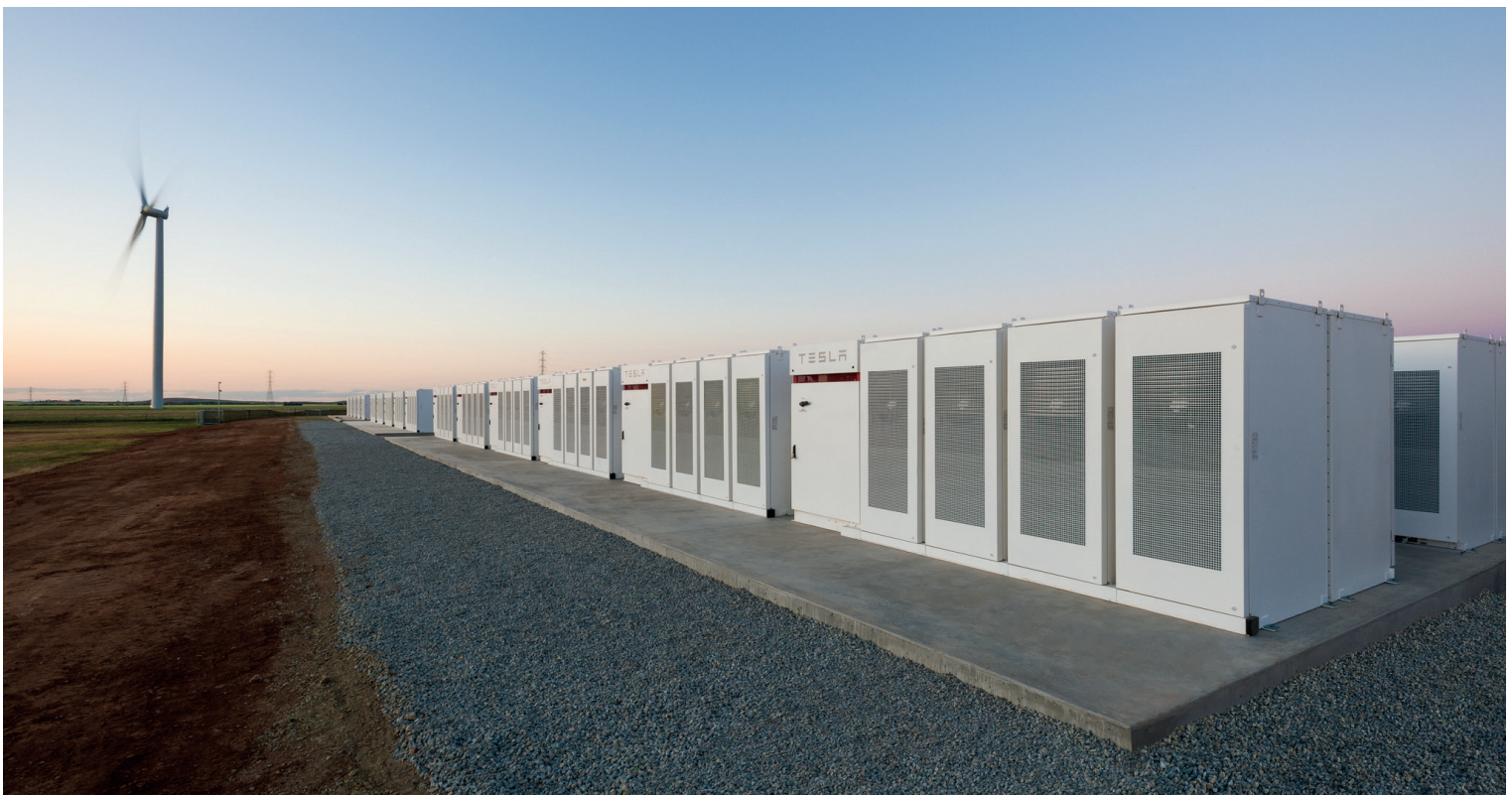
Figure 1: South Australia is in first place and is a global leader in transitioning to a grid with a high share of wind and solar backed by storage, thanks to projects such as the Hornsdale Wind Farm and Power Reserve.
