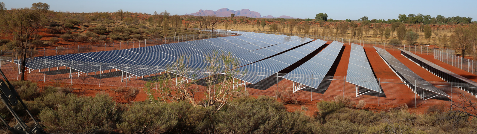
Figure 20: Yulara Solar Farm in the Northern Territory. Despite its significant solar resources, the Northern Territory has the lowest share of renewable energy of any state or territory.
