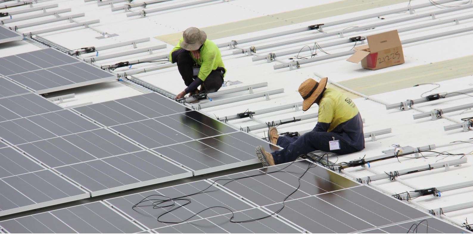
Figure 21: Workers install solar panels on a Logan City Council building, just south of Brisbane.
