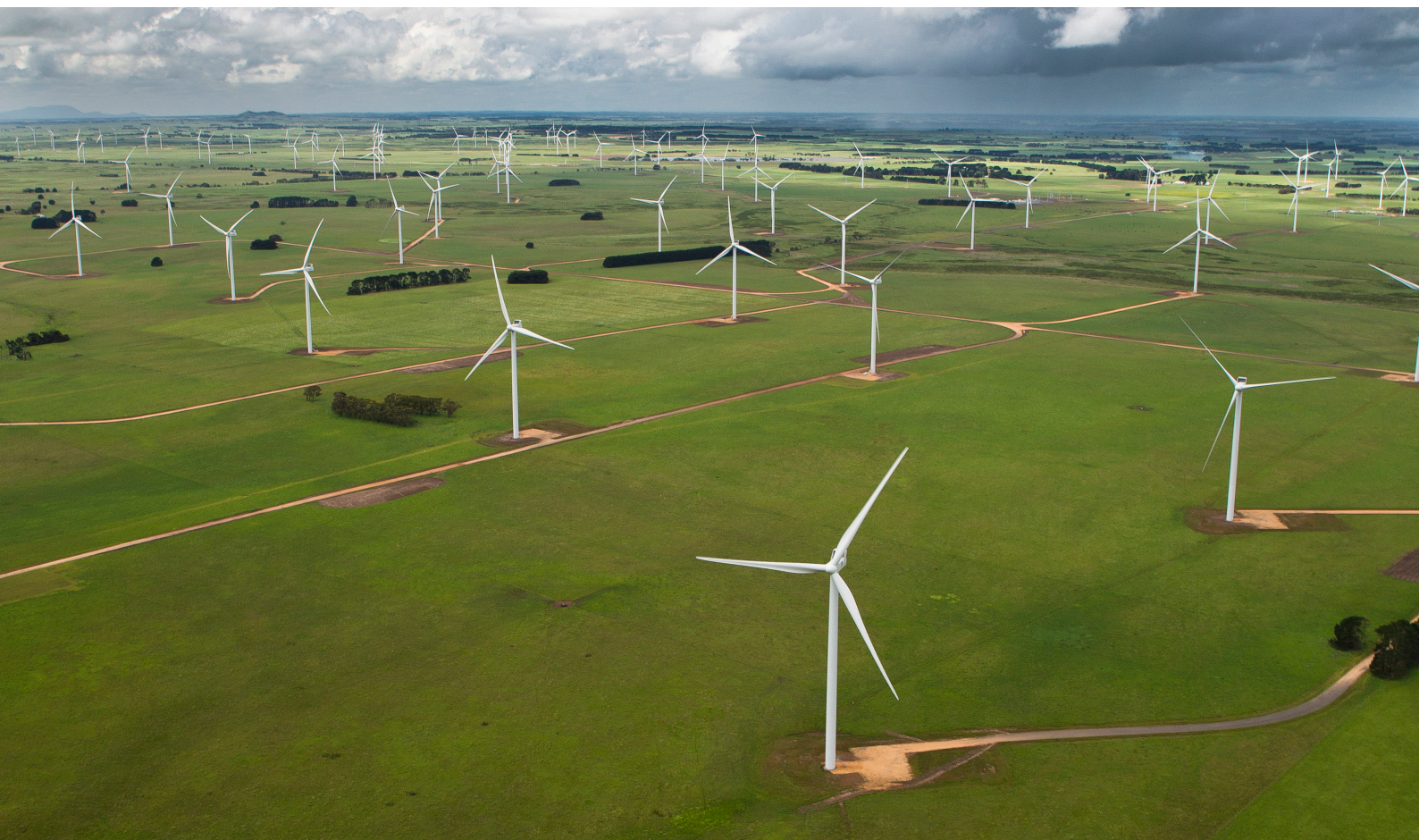
Figure 15: Victoria’s 420MW Macarthur Wind Farm. The state has a target of 50% renewable energy by 2030 and the most large-scale wind and solar capacity in the pipeline of any state or territory.
