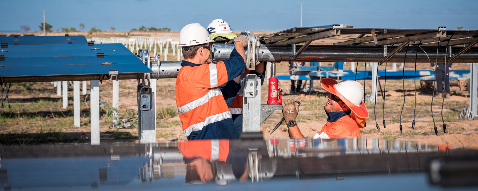
Figure 17: Workers install solar panels at the Kidston solar farm, intended to be integrated with the Kidston pumped hydro storage project in north Queensland.
