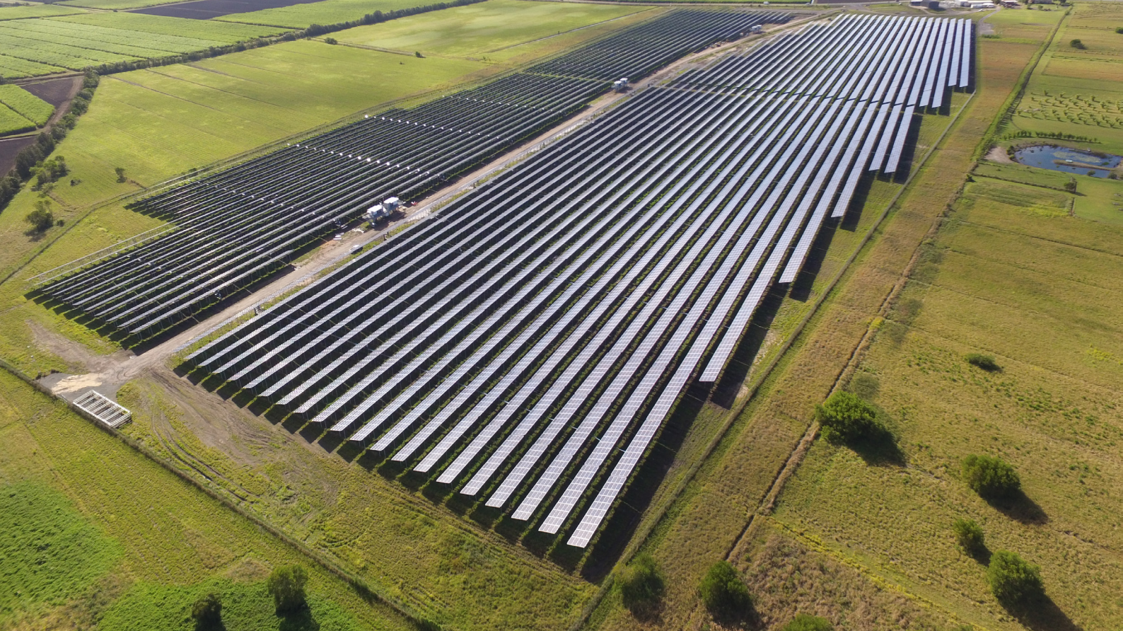
Figure 22: The 15MW Sunshine Coast Solar Farm, which offsets 100% of the electricity consumption of Sunshine Coast Council's facilities and operations.
