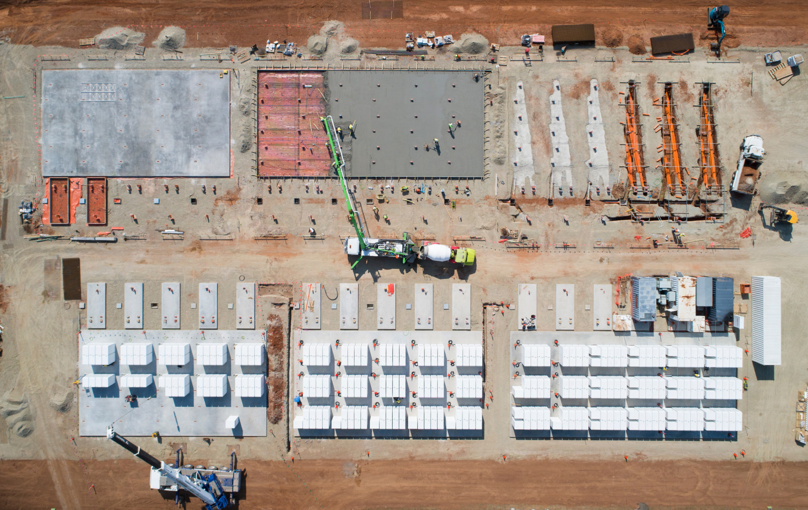
Figure 11: South Australia is balancing the complexities of a grid with high wind and solar penetration with storage projects, including the Tesla big battery at the Hornsdale Power Reserve.
