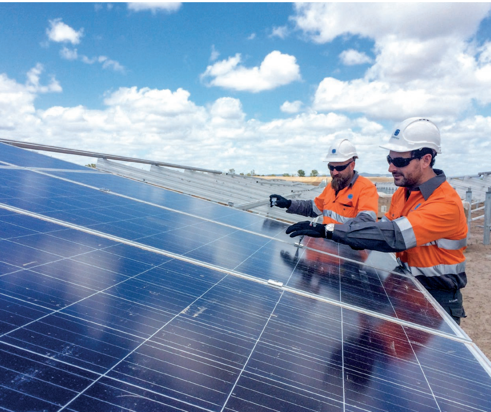
Figure 18: The Lakeland solar farm and storage facility (pictured) is now producing clean and affordable electricity and supporting jobs in the local area.
