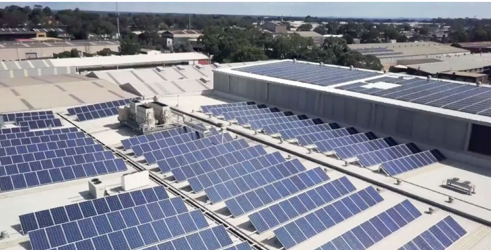
Figure 7: Households and businesses around Australia are installing rooftop solar to reduce their power bills. Bakers Maison has installed a 100kW rooftop solar system on its business in Sydney (pictured).
