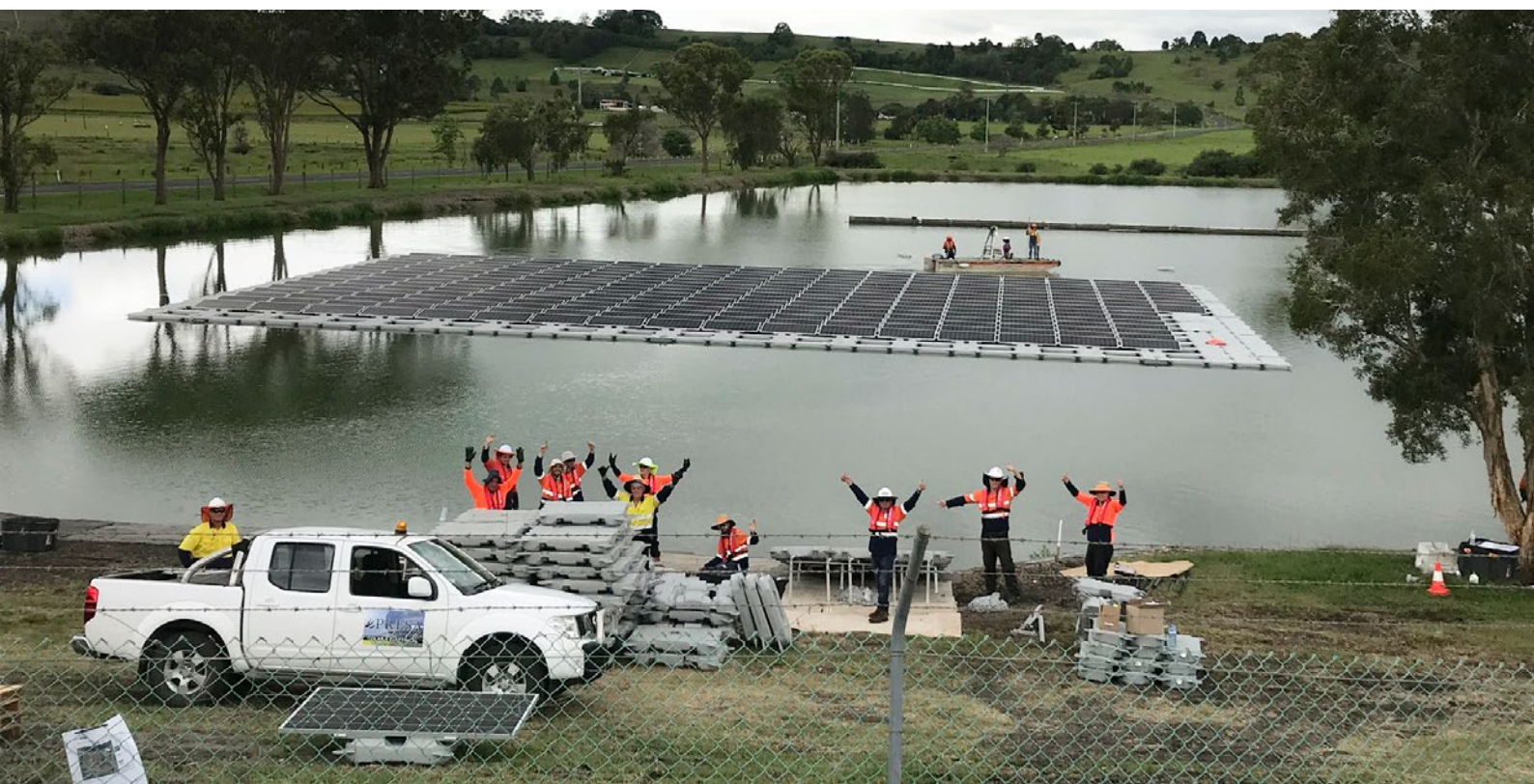
Figure 1: The 100kW Lismore floating solar farm, the largest to-date in Australia. Lismore City Council and other councils in New South Wales are backing renewable energy to help reduce their power bills and greenhouse gas pollution.
