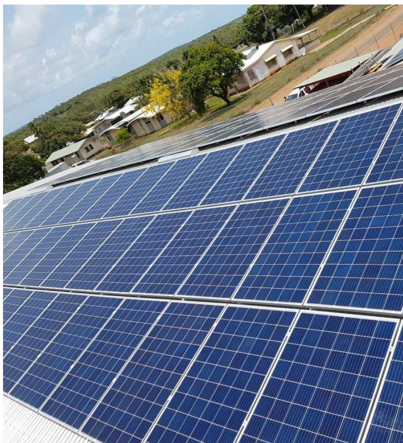
Figure 10: 750 solar panels have been installed in Lockhart River (below) to help reduce the community's energy bills.
