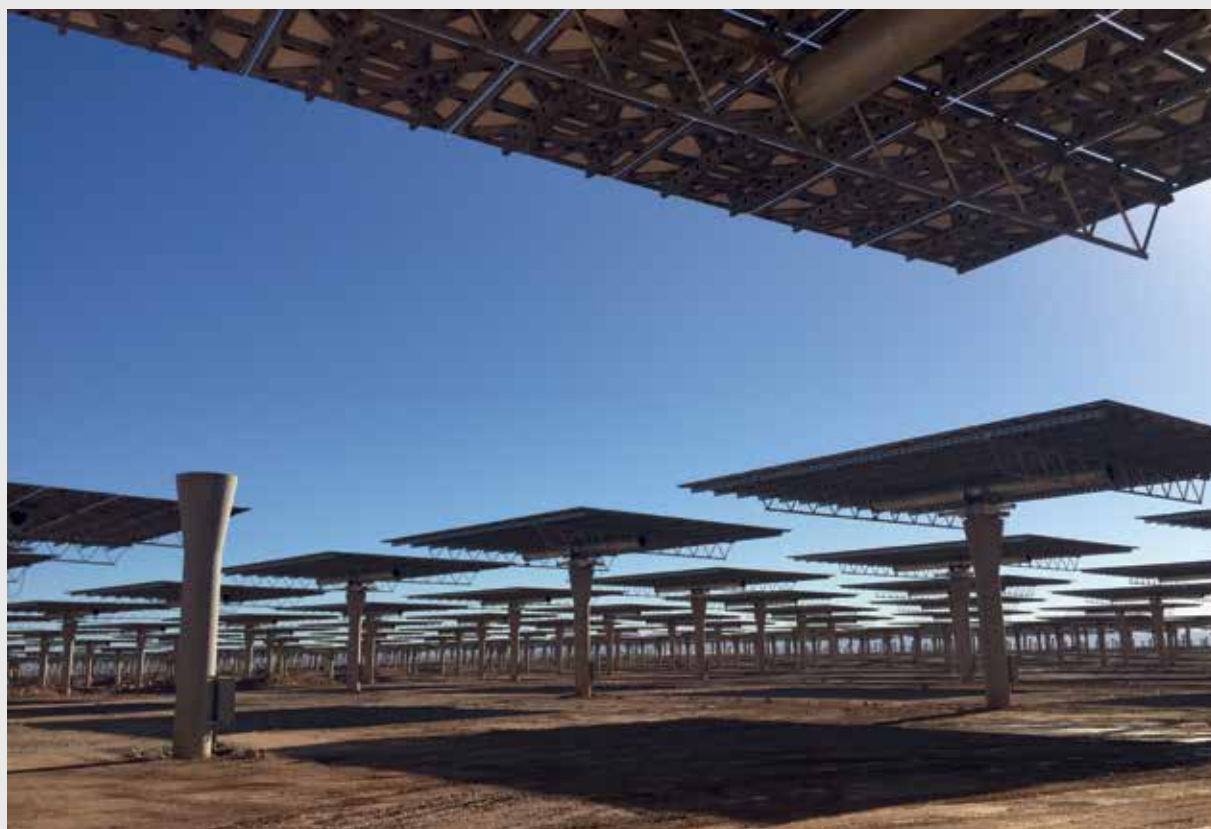
Figure 7: Morocco's Noor-Ouarzazate Solar complex.
