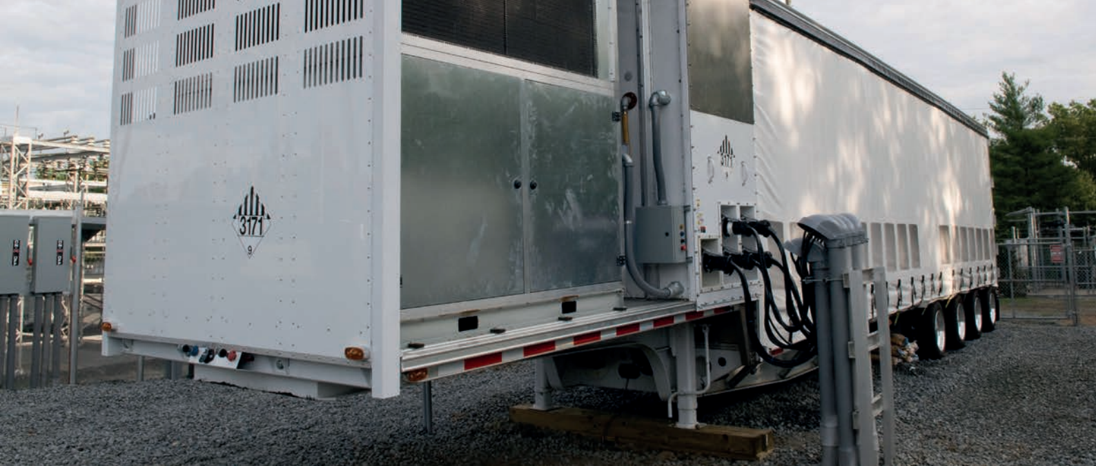
Figure 17: Large battery for network use.
