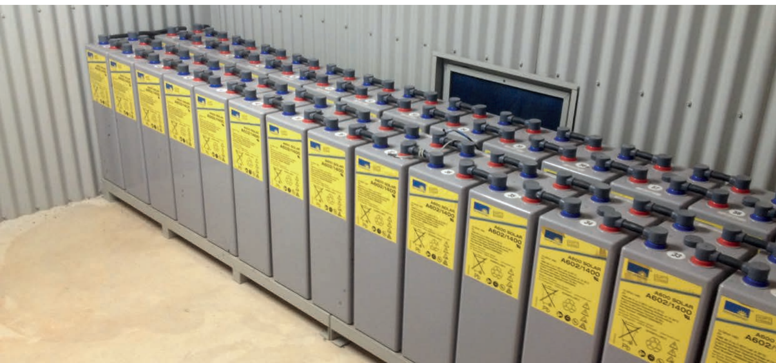
Figure 14: Off-grid battery bank for solar PV in Western Australia.
