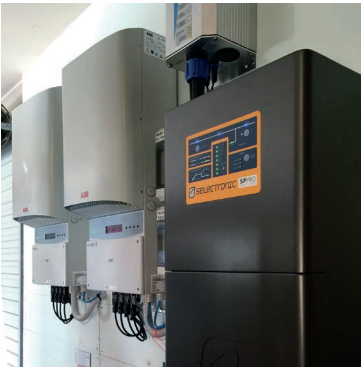
Figure 8: An example of a household solar pv battery storage system.
