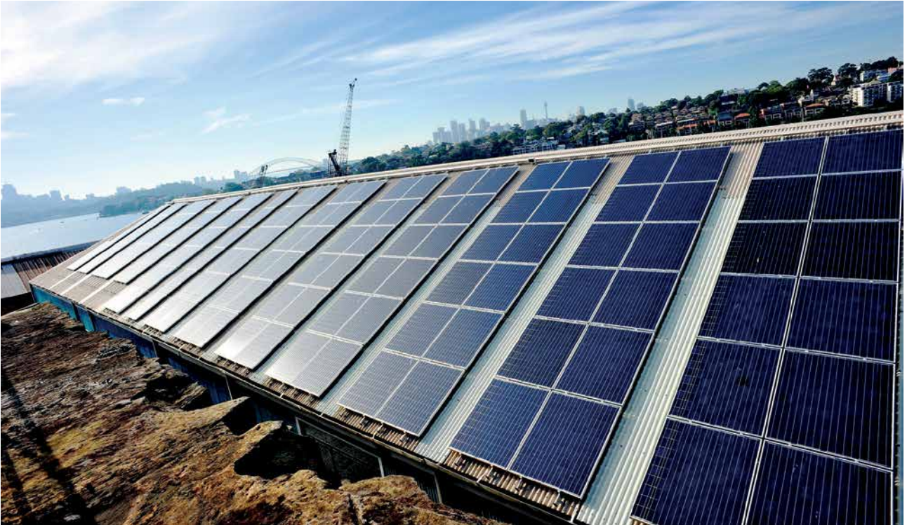
Figure 12: Solar Panels in Sydney.
