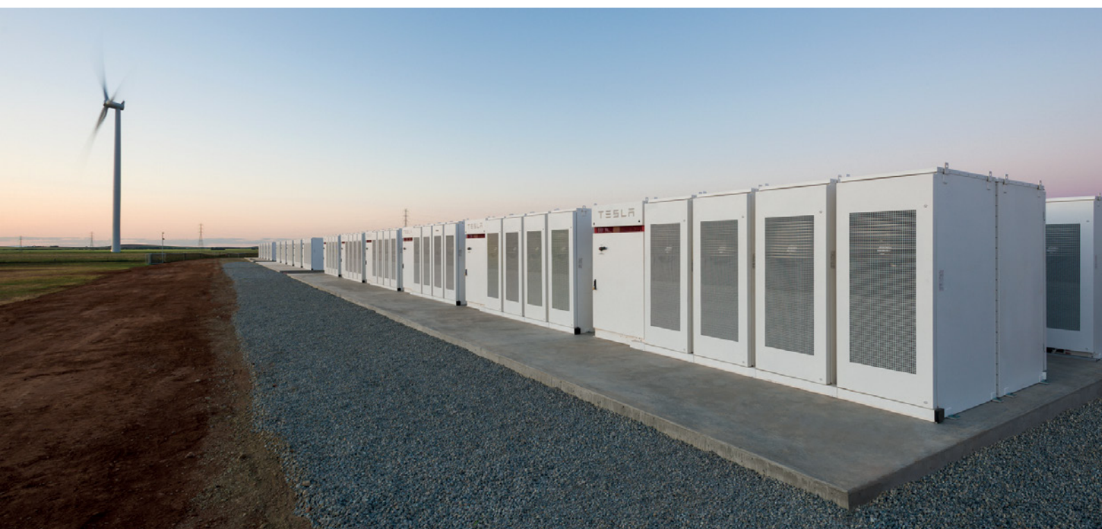
Figure 2: South Australia's Hornsdale Power Reserve.
