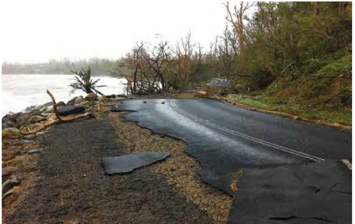
Figure 12: An example of damage to a road from coastal flooding.
